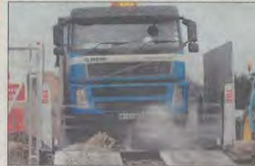
CLEAN MACHINE: A HGV taking mud from Badnells Pit has its wheels washed before leaving the site. Ref:108609-39
